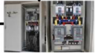
Electric panel board
